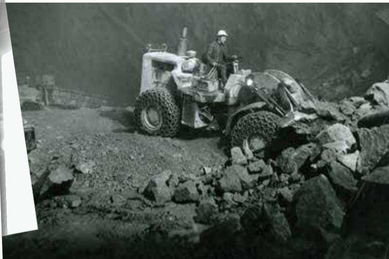
Excavation work being carried out on the massive engineering project which commenced in 1968.
