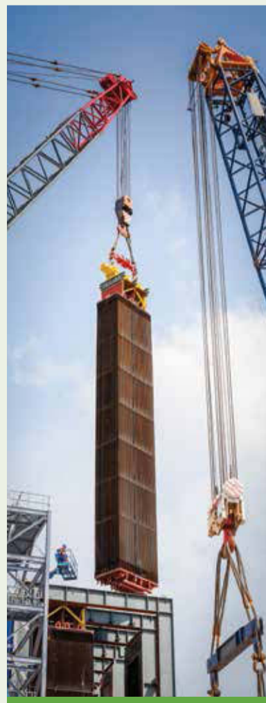
Heat exchange module, mid manoeuvre.
