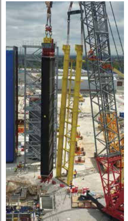
The first heat recovery steam generator (HRSG) boiler module was installed at Carrington power plant during April.
