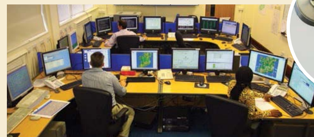
Telecoms Operations Centre.
